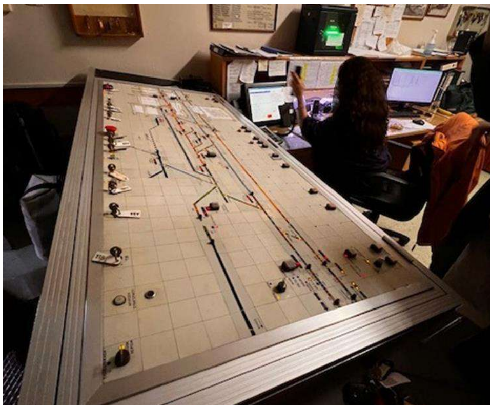
Figure 41. Positions of station masters when facing the control panel (above) and when communicating (below) in Larissa station.
